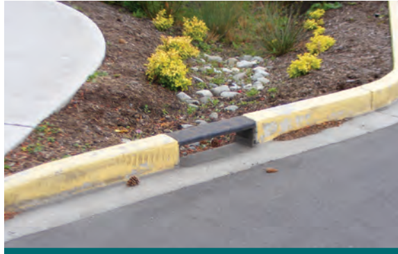
Figure 6.4.4: A covered curb cut can be used to provide the protection of a curb but allow runoff to enter the facility. (Source: Aquafor Beech)
