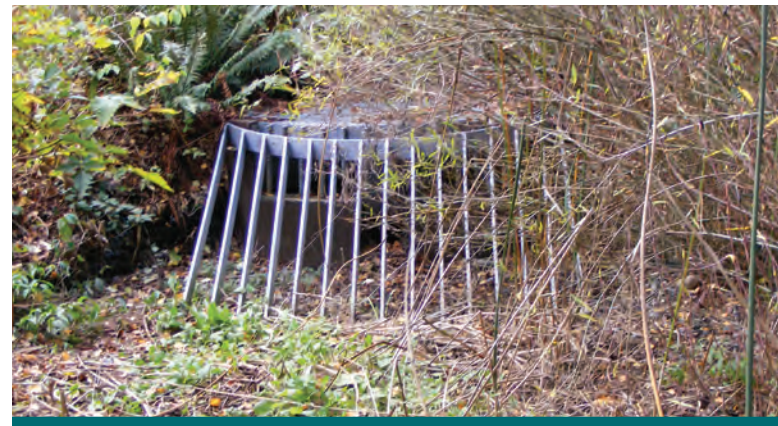
Figure 6.4.10: Overflow grate inverts should be surveyed to confirm that they will function as intended during infrequent storm events. Vegetation should be managed around overflow grate inverts to prevent clogging. (Source: Aquafor Beech)
