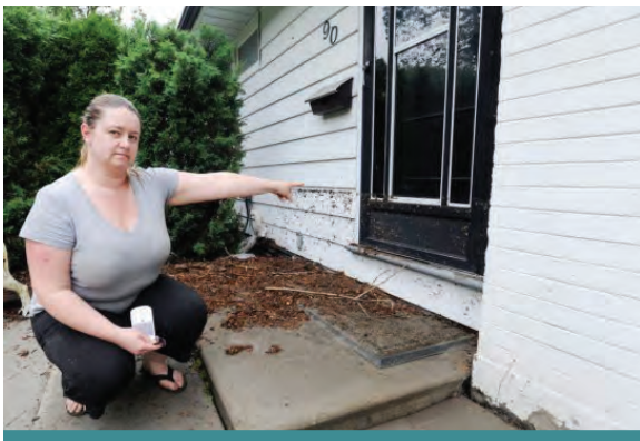
Figure 1.1.1: July 8, 2013 flooding also impacted private property. In this photograph a Mississauga resident shows the structural damage that took place to her home. (Source: Fred Loek, Mississauga News)
