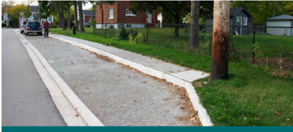
Figure 2.5.3: Pervious concrete requires a modified poring and setting approach when compared to standard concrete. Porous concrete was used to create a permeable parking lay-by in Streetsville in Mississauga. (Source: CVC)
