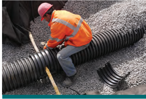
Figure 9.4.6: The next step was placing a piece of perforated pipe on top of the gas line to prevent blockages in the pipe when the trench was filled with clear stone. (Source: Aquafor Beech)
