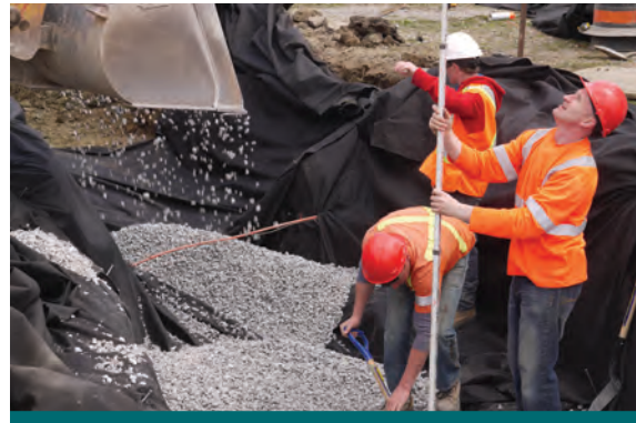
Figure 9.2.2: Contractors verifying the location and elevation of bioretention planters during construction at the Elm Drive Project. (Source: CVC)
