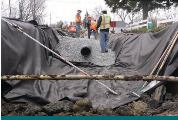
Figure 9.4.4: At the Lakeview Project a gas line was found to span the bioswale trench. Moving the gas line was not an option. An adaptive approach using avoidance was determined to be the best course of action. (Source: Aquafor Beech)
