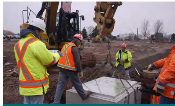
Figure 2.4.7: To maximize treatment and water balance benefits, proprietary stormwater treatment devices can be installed upstream of LID practices. (Source: CVC)
