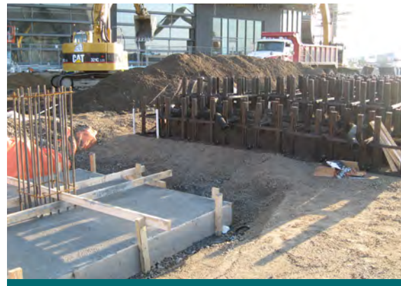
Figure 10.2.3: Proper installation of soil support systems ensures settling does not occur and maintenance is not required. (Source: Deep Root.)
