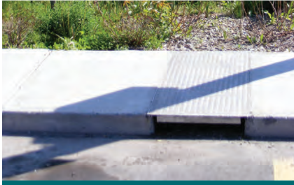
Figure 6.4.2: Ensure that grates are corrosion resistant and have anti-slip measures. (Source: Aquafor Beech)
