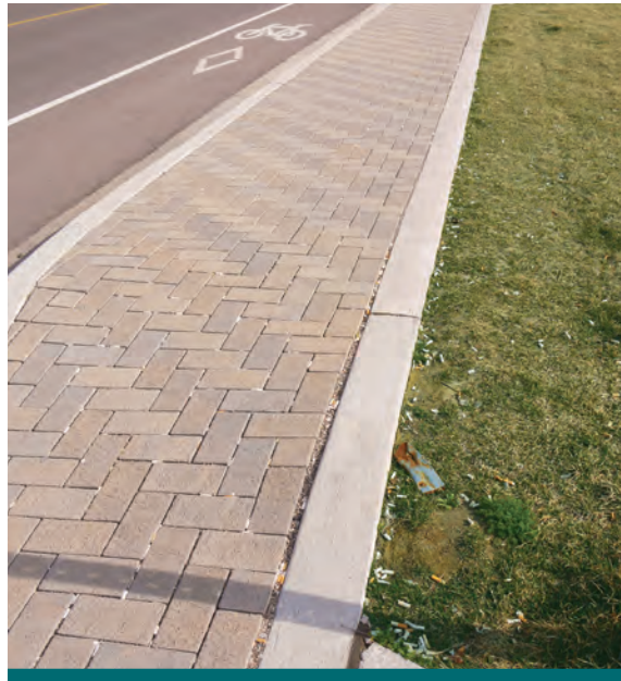
Figure 4.3.34: Further consideration of user behavior may have resulted in a different LID solution for this location. This section of sidewalk is a preferred smoking location for the adjacent business and the cigarette butt waste stuck between the permeable pavers will be an ongoing maintenance problem. (Source: CVC)
