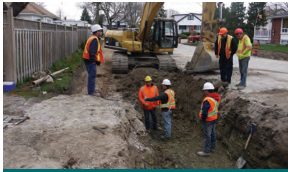
Figure 9.2.3: During the construction of the Lakeview Project the bioswale trench alignment travelled off-centre due to over-excavation. The team lead used the passive approach since the excavation could not be reinstated and the error did not cause negative impacts to the design. (Source: Aquafor Beech)
