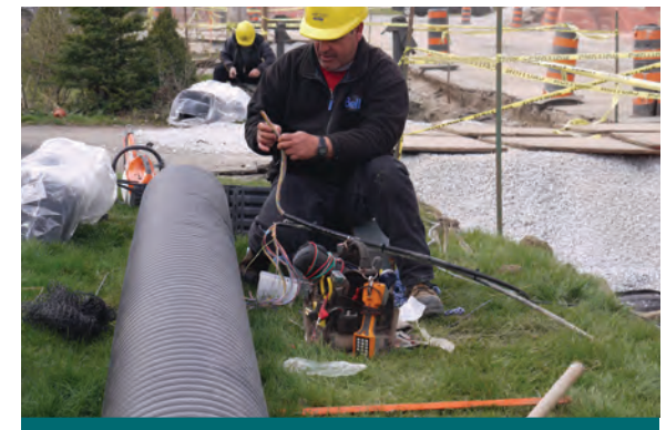
Figure 9.4.3: When utilities are damaged, expect additional people onsite. In this photo communications technicians establish service after damage to a cable at the Lakeview Project. (Source: Aquafor Beech)
