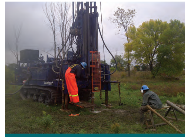
Figure 5.2.1: Before undertaking a geotechnical investigation, consider what equipment will be required. Where large equipment such as a drill rigs is required it is essential to ensure there is a safe ingress and egress for all equipment and people. Also consider how the work will affect user of the ROW and adjacent properties. Traffic controls may be required on confined or busy roads. (Source: Aquafor Beech)
