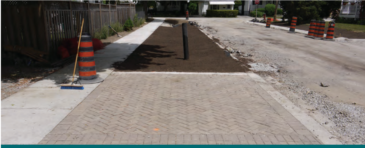
Figure 9.3.1: Construction activities including excavation, sawing, and delivery of materials can cause debris and sediment deposition across a construction site even during good weather. It is essential that bioretention soil media is not delivered and installed until the surrounding area is clean. (Source: Aquafor Beech)
