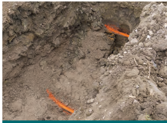
Figure 9.4.1: To prevent damage to pipelines and utilities, daylighting is done prior to excavation with heavy machinery in the vicinity of the utility locate. In this photo utilities are marked with orange paint after being exposed. (Source: Aquafor Beech)
