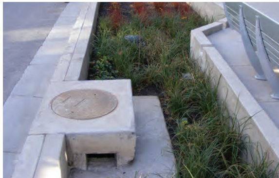
Figure 6.4.5: Inlets and outlets can be incorporated into a manhole by controlling the stage-discharge characteristics with an orifice plate or weir. (Source: Aquafor Beech)
