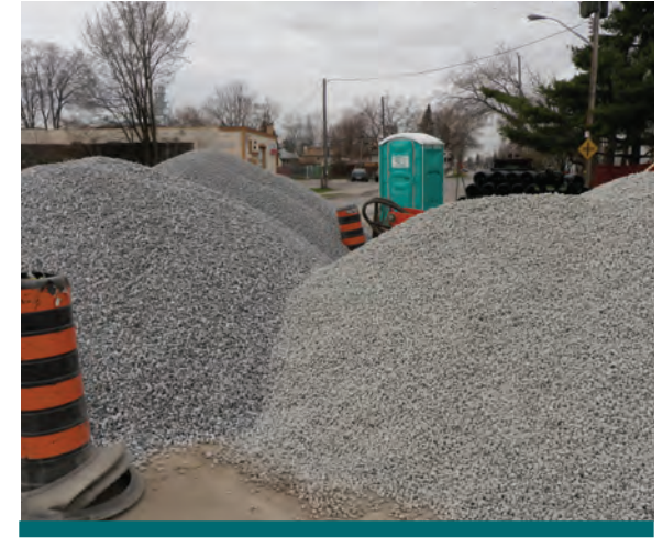
Figure 9.3.2: To the untrained eye both stockpiles of clear stone look similar. An experienced construction supervisor would be able to differentiate the single-washed stone on the right from the double washed on the left. In this case, double washed stone was specified to prevent clogging of the system with stone dust. (Source: Aquafor Beech)
