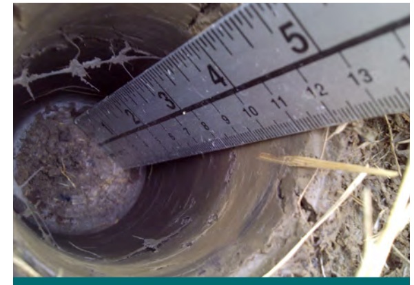
Figure 10.3.2: Coring has indicated that a layer of impermeable clay has clogged this bioretention unit. Major rehabilitation including replacement of the bioretention soil media will be required to allow for filtration and infiltration. (Source: Aquafor Beech)
