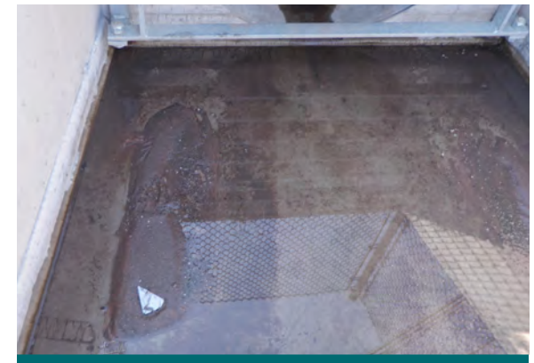
Figure 10.2.4: Along with measuring sediment depth in a proprietary stormwater treatment device, check the outlet structure if accessible. If the OGS is functioning as intended, sedimentation should not be occurring. (Source: Aquafor Beech)
