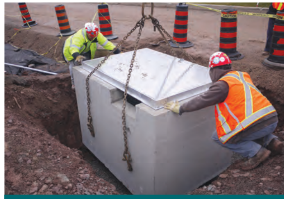
Figure 4.3.15: Prefabricated modules can be used on local industrial roads to capture high sediment loads. (Source: CVC)
