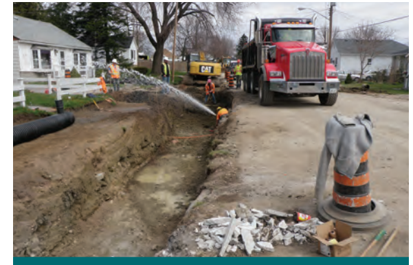
Figure 9.4.2: The costs associated with damage to a pipeline or utility will depend on the type of utility and may include response, repair, environmental impact mitigation measures, and restoration. (Source: Aquafor Beech)
