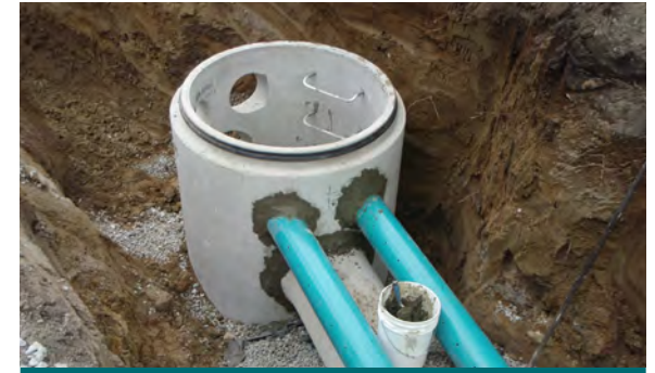
Figure 2.3.1: Perforated pipe systems employ many of the same materials and construction practices as conventional storm sewer pipes, instead using perforated pipes to encourage infiltration during conveyance. (Source: Aquafor Beech)
