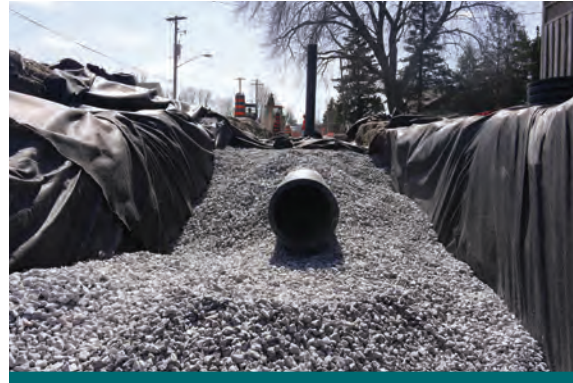
Figure 9.2.1: On-site construction supervisors can verify design elements as they are being built. This perforated pipe will soon be buried. Verifying pipe size, invert elevation, and trench dimensions must occur before the trench is filled. (Source: Aquafor Beech)
