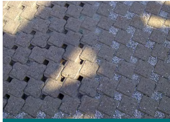
Figure 10.3.3: In this photo the aggregate has been removed from permeable interlocking concrete pavers. This will need to be replenished immediately to avoid clogging of the joints. (Source: Aquafor Beech)
