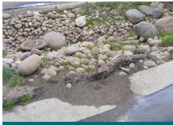
Figure 10.3.1: Failure of sedimentation and erosion controls may cause significant impairments to infiltration practices. In this instance, wait until construction has finished before rehabilitating bioretention area. (Source: Aquafor Beech)
