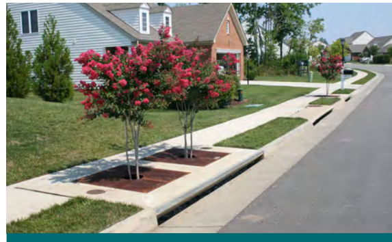
Figure 2.4.1: A Filterra Bioretention System (the flowering plantings and buried precast unit pictured above) is one type of precast tree planter. (Source: Filterra Bioretention Systems)
