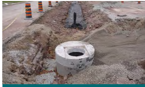
Figure 6.14.1: At the Elm Drive project, the design included a manhole for the collection of water quantity and quality samples, located downstream of the LID practices. (Source: CVC)
