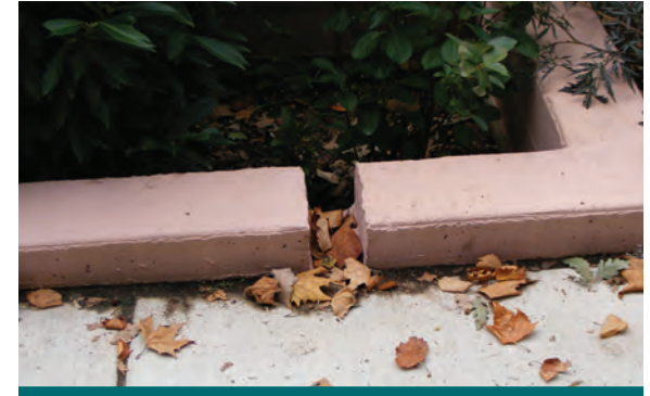
Figure 6.4.6: Notched curb cuts prevent larger debris from accumulating in bioretention planters. A greater number of curb cuts may be required to allow for design flow conveyance. (Source: Aquafor Beech)
