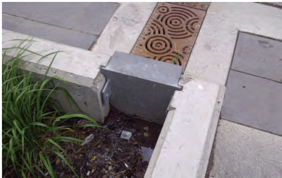
Figure 6.4.3: The gates on this bioretention planter in Kitchener, Ontario are designed to close during the winter season to prevent infiltration of chloride from deicing practices. (Source: Aquafor Beech)
