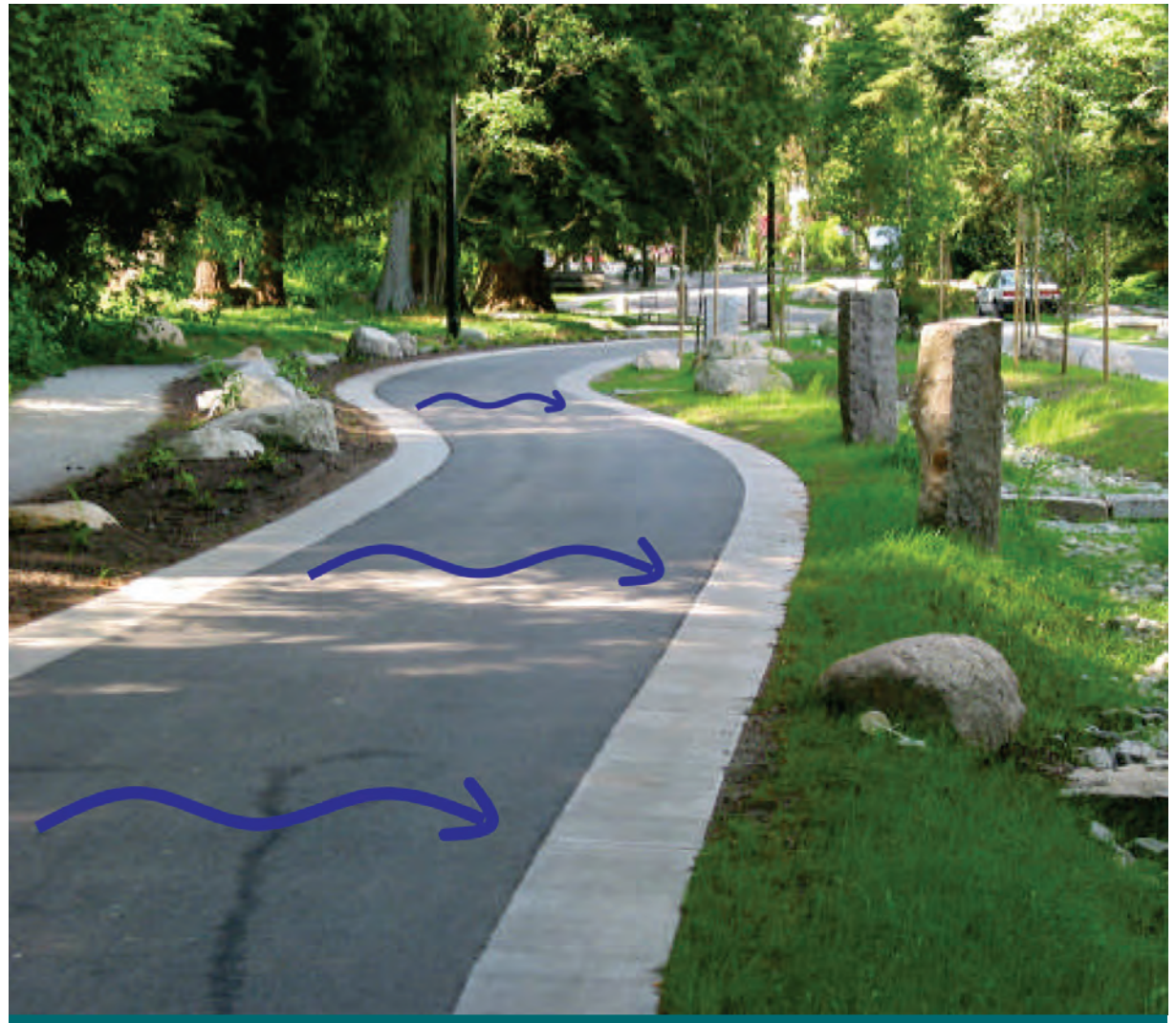
Figure 6.4.1: Flush curbs on both sides of this street allow for drainage from left to the bioswale on the right. (Source: City of Vancouver)
