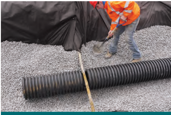
Figure 9.4.5: The above photo shows how the perforated pipe was installed around the exposed gas line at the Lakeview Project. A notch was cut in the perforated pipe and fit into place below the gas line. (Source: Aquafor Beech)
